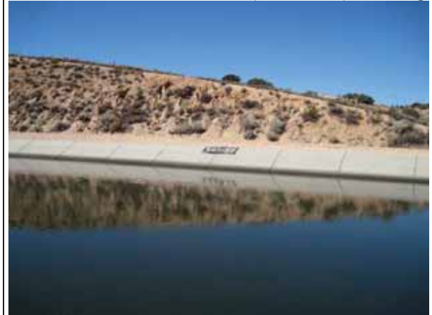
08/06/12, Camera A2 Frame 1027: Numbers visible on west side of canal wall.
