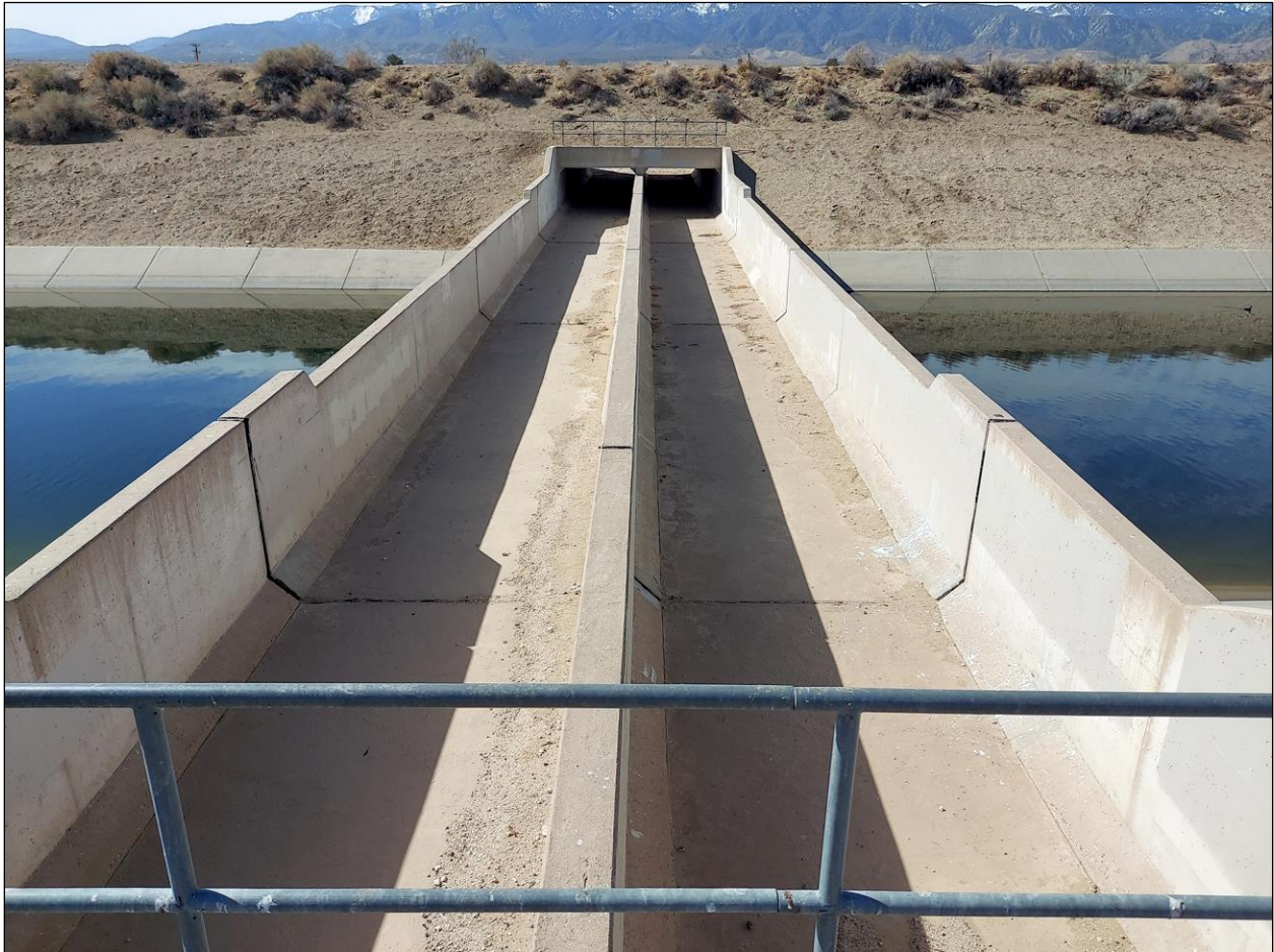
Figure 10. Portion of the California Aqueduct in the project area. (Photograph taken on March 25, 2021; view to the south)
